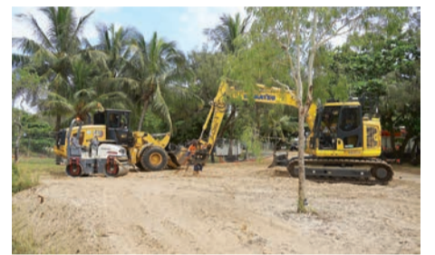
Construction is underway on the Great Keppel Island (Woppa) Arrivals Plaza, set to transform the visitor experience at Fishermen's Beach.
