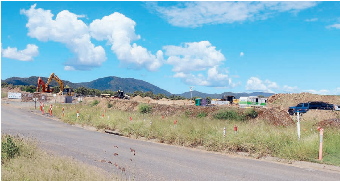
Works are already underway on site for BMD Bielby RRR Joint Venture LTD's precast yard. (Matthew Pearce: 543513)
