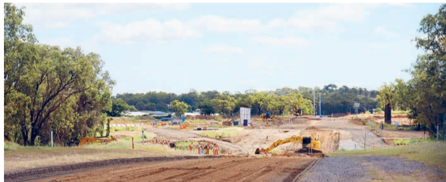
Work on the Rockhampton Ring Road is underway at Alexandra St, Parkhurst near the planned new Fitzroy River crossing. (Matthew Pearce: 545341)
