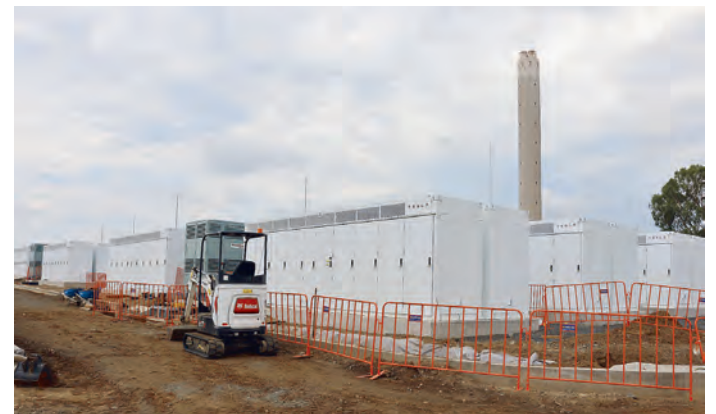
Some of batteries behind Stanwell Power Station.
