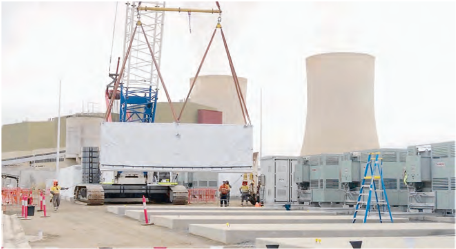
One of the final Megapack units being delivered at the Stanwell Battery site. (Supplied)
