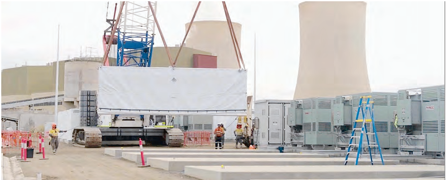
One of the final Megapack units being delivered at the Stanwell Battery site. (Supplied)
