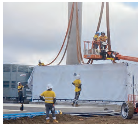
The first consignment of Tesla Megapack 2XL units arrived at the project site adjacent to Stanwell Power Station last month. (Supplied)
