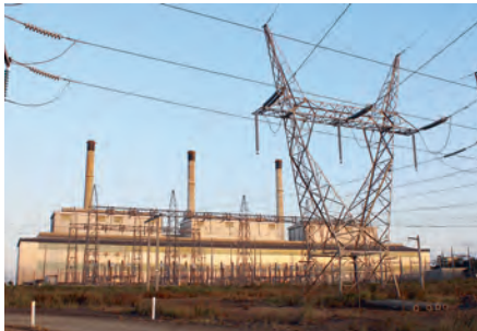
Rio Tinto holds a 42.125 per cent in the NRG Gladstone power station, scheduled to close in 2035. (File)
