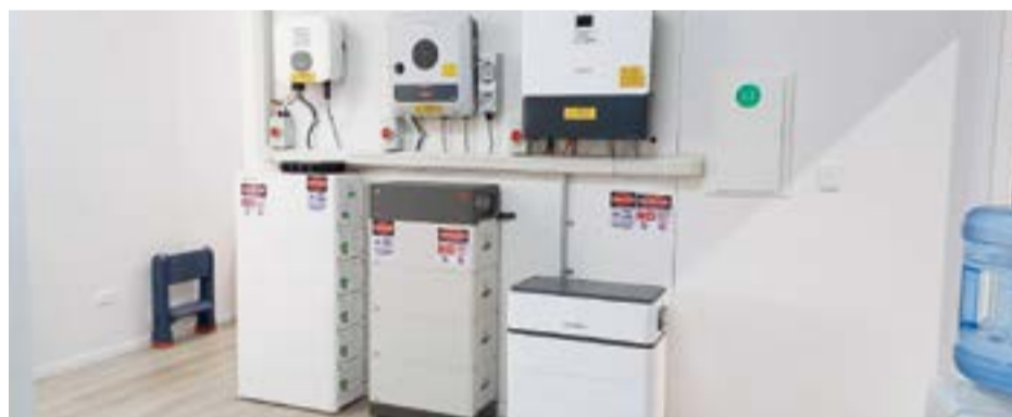
The innovative battery system and inverter display.
